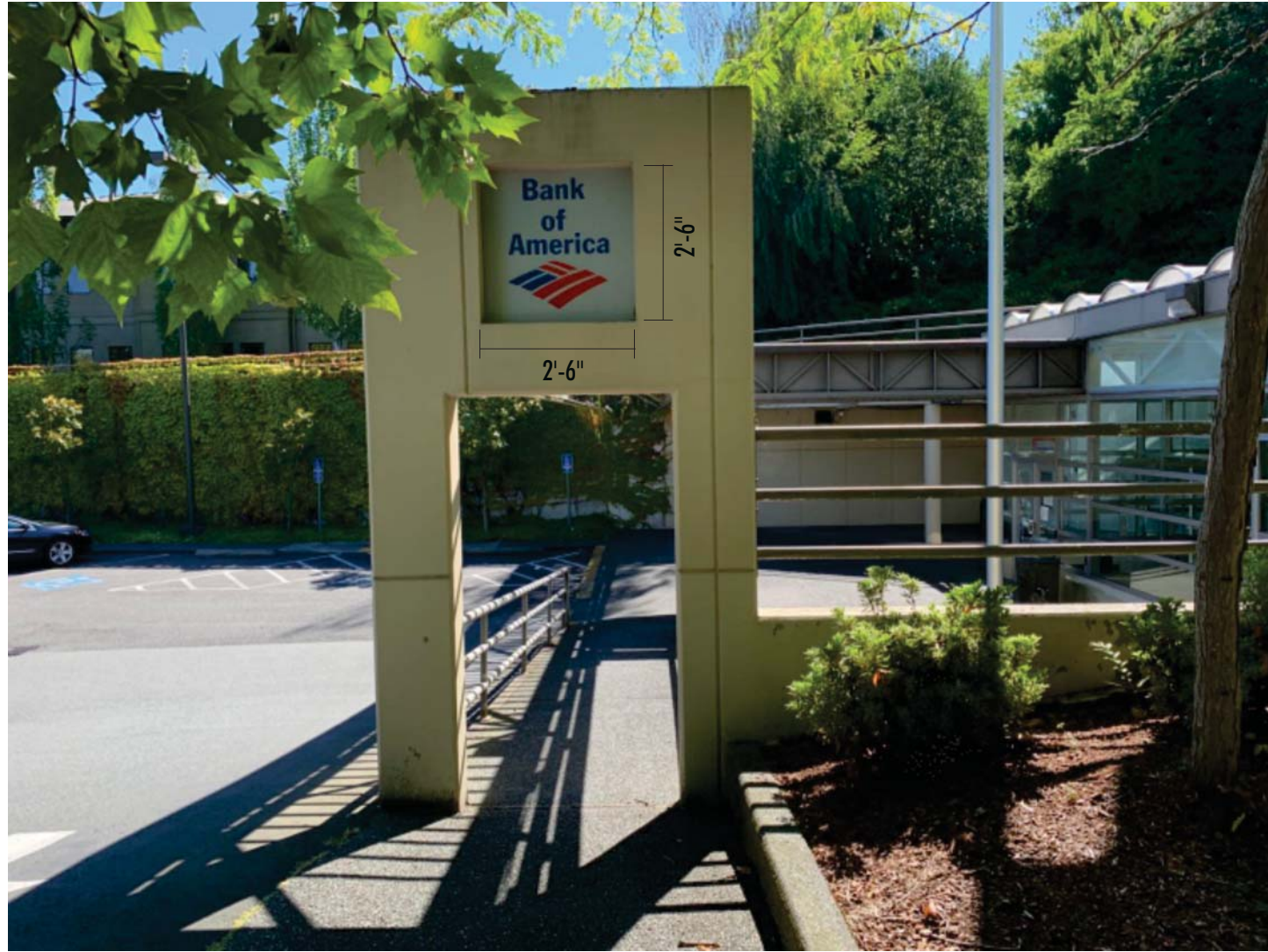
EXISTING SIGNAGE | PANEL TO BE REMOVED & DISCARDED | PATCH & PAINT HOLES T/M FASCIA COLOR
