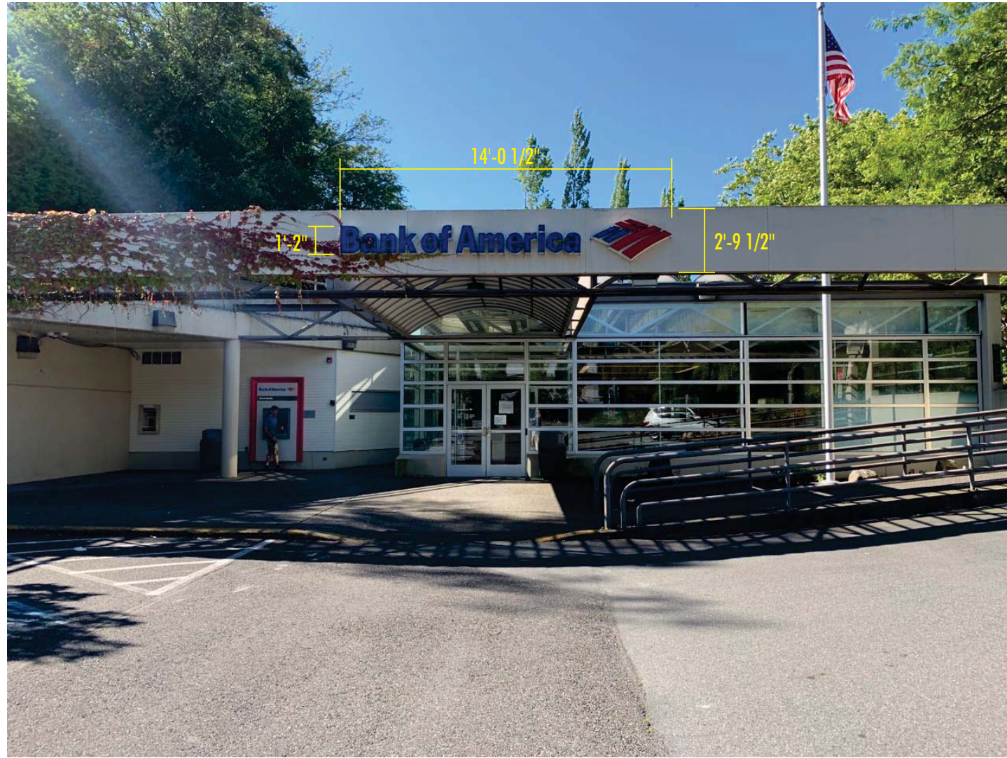
EXISTING SIGNAGE | TO BE REMOVED & DISCARDED | PATCH & PAINT HOLES T/M FASCIA COLOR
